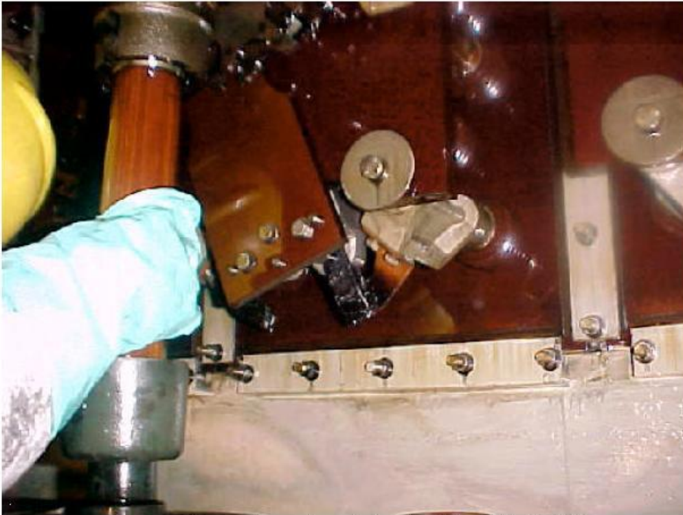
Damaged reversing switch contacts Phase B in the LTC FIGURE 1
