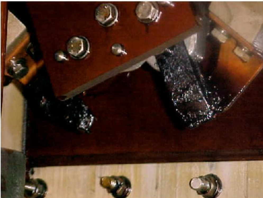
Close-up view of the damaged reversing switch contacts FIGURE 2
