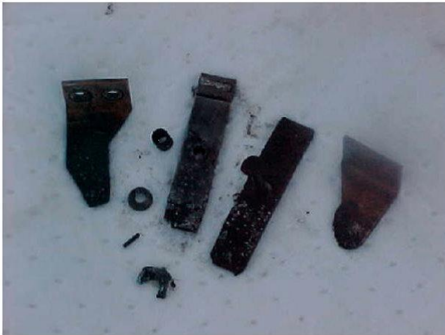
Damaged contacts on Phase B reversing switch FIGURE 3
