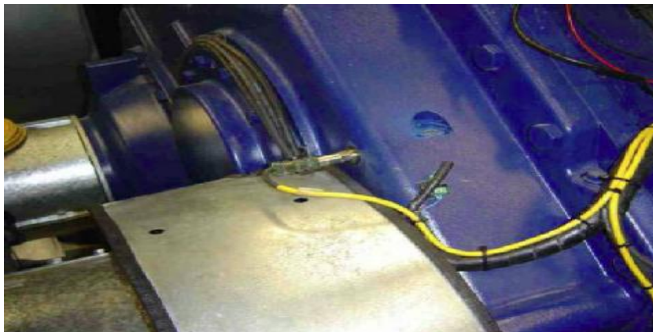
PMS gearbox accelerometers
